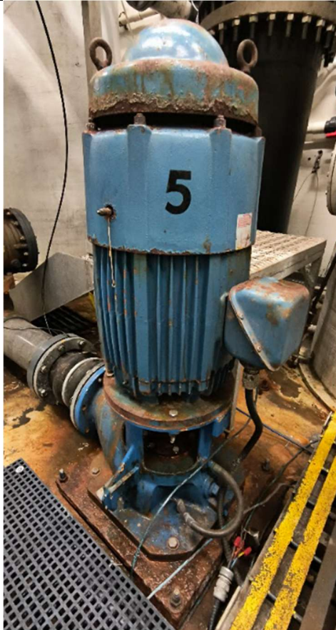
Image 3. LSS 5 a 40hp Goulds VIT pump is the last supply pump awaiting rebuild.
