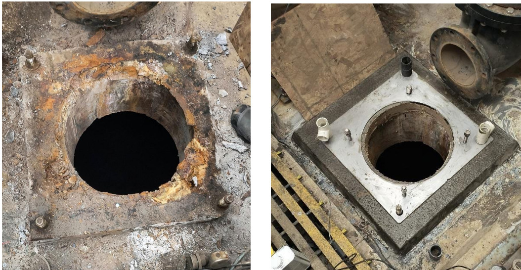
Image 1. Condition of grout after removal of bedplate shown (left) and after replacement bedplate installed and precision leveled in new grout (right).
