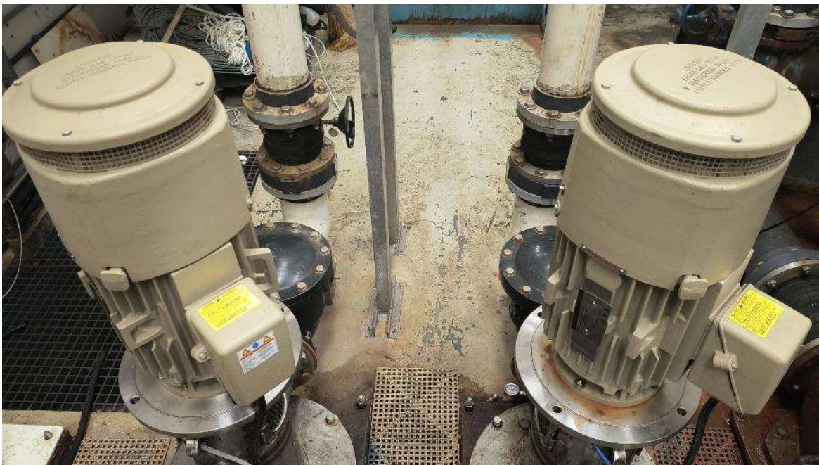
Image 6. Newly installed pumps LSS-6 and LSS-7 provide for greater efficiency and bring critical water systems back into design operating pressures,
