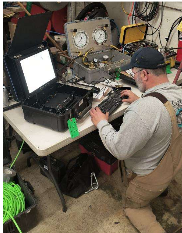
Image 2. American Marine foreman monitors equipment and diver in the intake well performing dredging operation.
