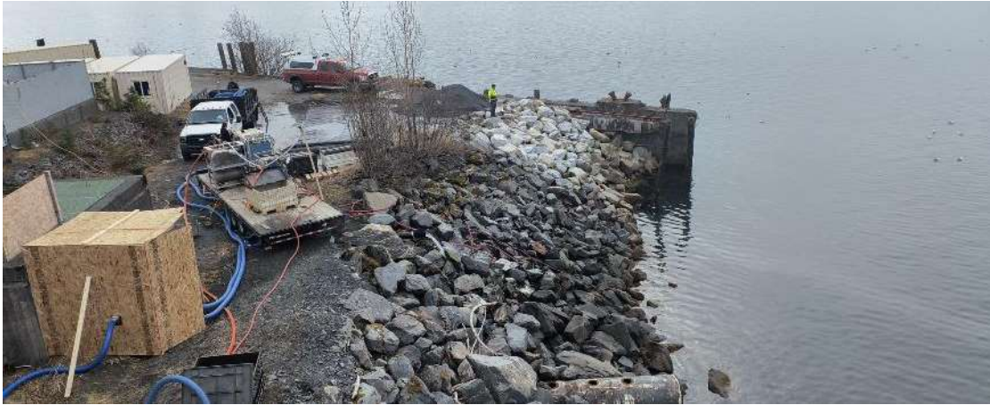
Image 3. PND Engineer (center, in high vis jacket) monitors runoff water from dredging operation ensuring compliance with USACE permit and the performance of the sediment collection bags. A plywood enclosure was constructed around a large diesel pump to reduce noise exposure for ice seal and common murre habitats.
