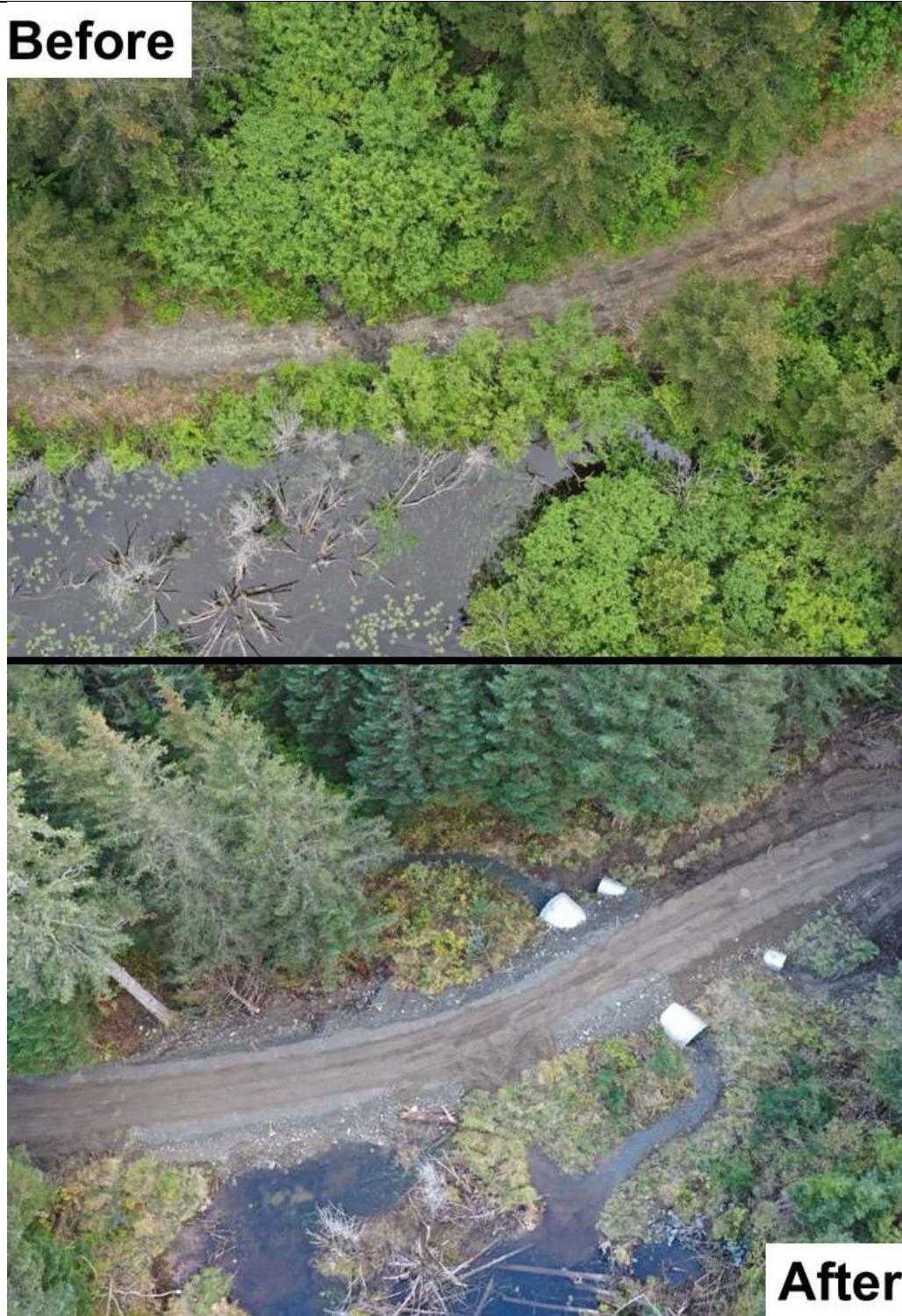
Figure 1. A before and after comparison photo of the Windy Bay culvert replacement project.
