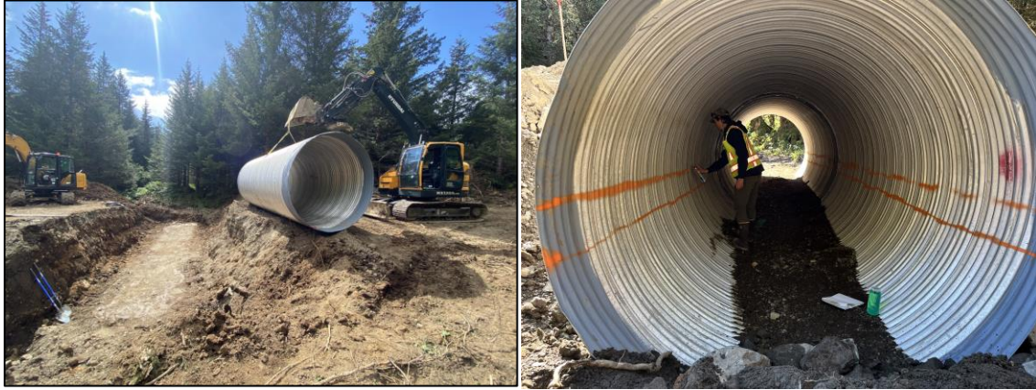
Figure 2. Photos of the Windy Bay Culvert removal site in Q2, 2024. The photo on the left depicts the culvert pipe prior to placement at grade. The photo on the right depicts painting the culvert infill elevation lines in the culvert.
