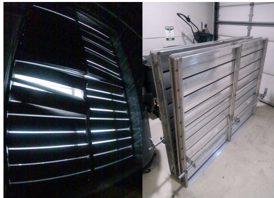
Image 1. New AHU-6 relief dampers (right) replacing failed dampers (left)
