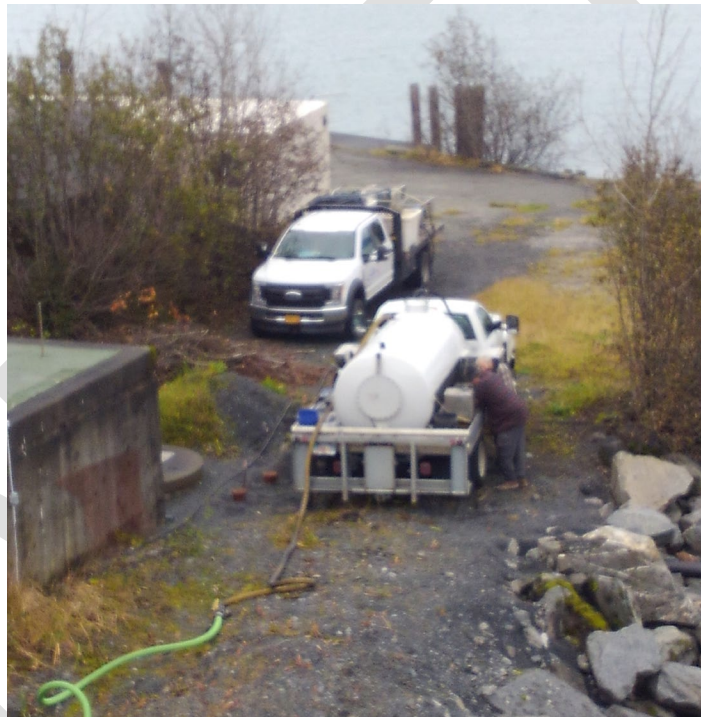
Suction equipment used to support initial dive and inspection of intake wells.
