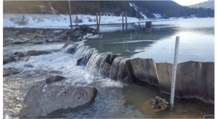
Photo 2. A look across the weir at the perch and water surface drop. This also shows where the recent displacement of the weir occurred, moving the sheet pile downstream 5-6 feet (USFS 2020).
