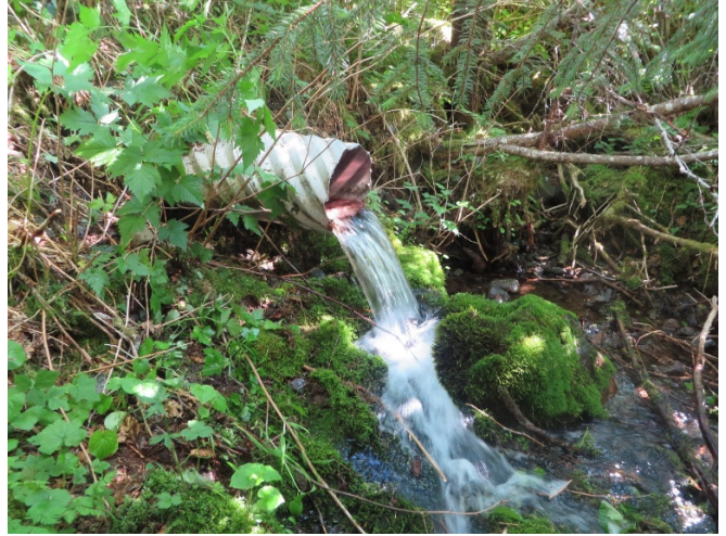
Figure 5. AKSF # KAC01-155. Perched culvert functions as full barrier for resident fish on unnamed stream.
