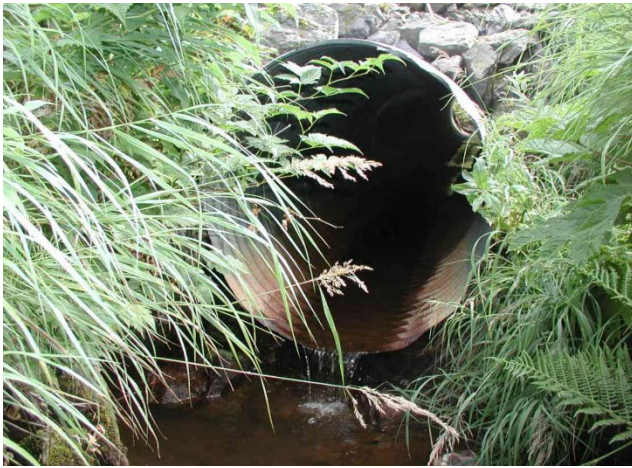
Figure 6. ADF&G 20300918. Perched and twisted culvert restricts upstream movement of juvenile salmon.
