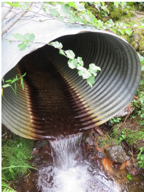
Figure 2. ADF&G #20300915. Perched culvert preventing upstream fish passage
