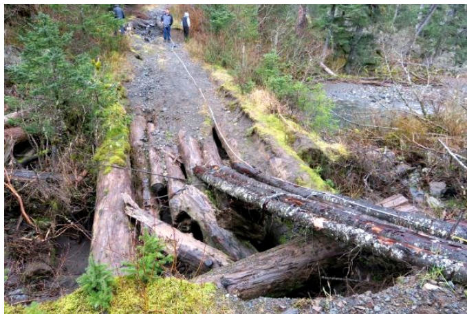
Figure 3. AKSF #01B15. This crossing will be replaced a bridge using TTP funds secured by the Port Graham Village Tribe.
