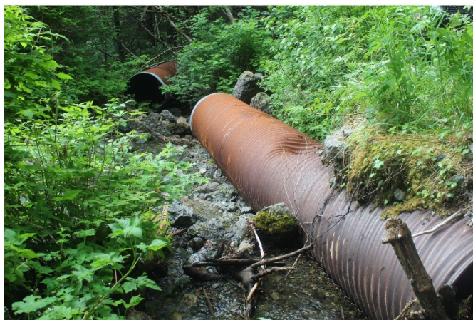
Figure 4. PGC # 004. Failed culvert on main road to Rocky Bay
