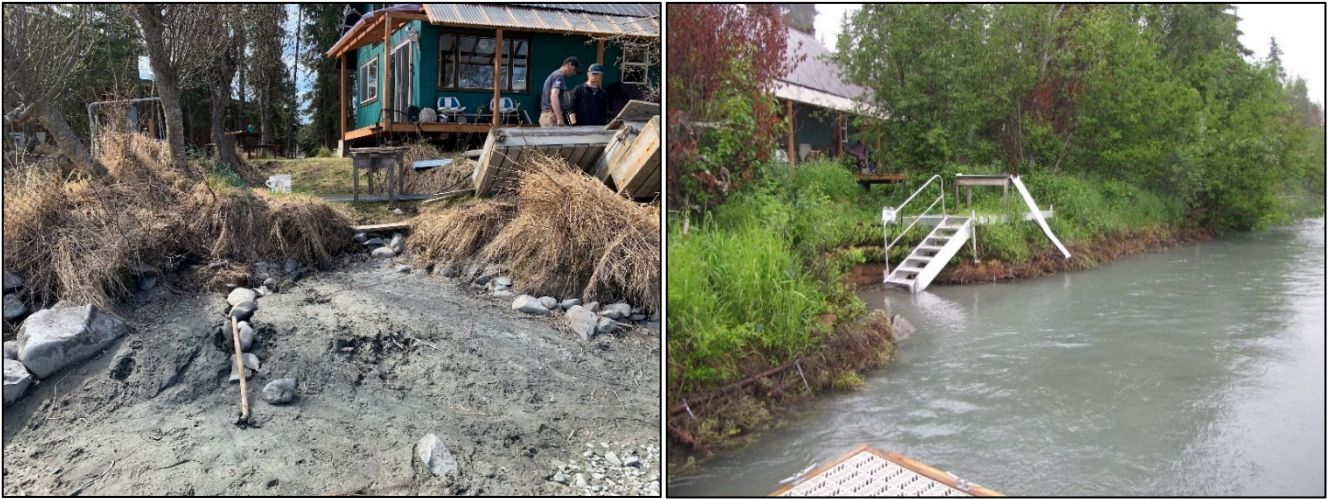
Figure 3. Picture on left, prior to construction 2020, shows damage caused by people entering the river to fish. Photo on the right, after construction 2020, shows a completed project with 2 brush layers an elevated light penetrating walkway (ELP) and staircase for people to enter the water.
