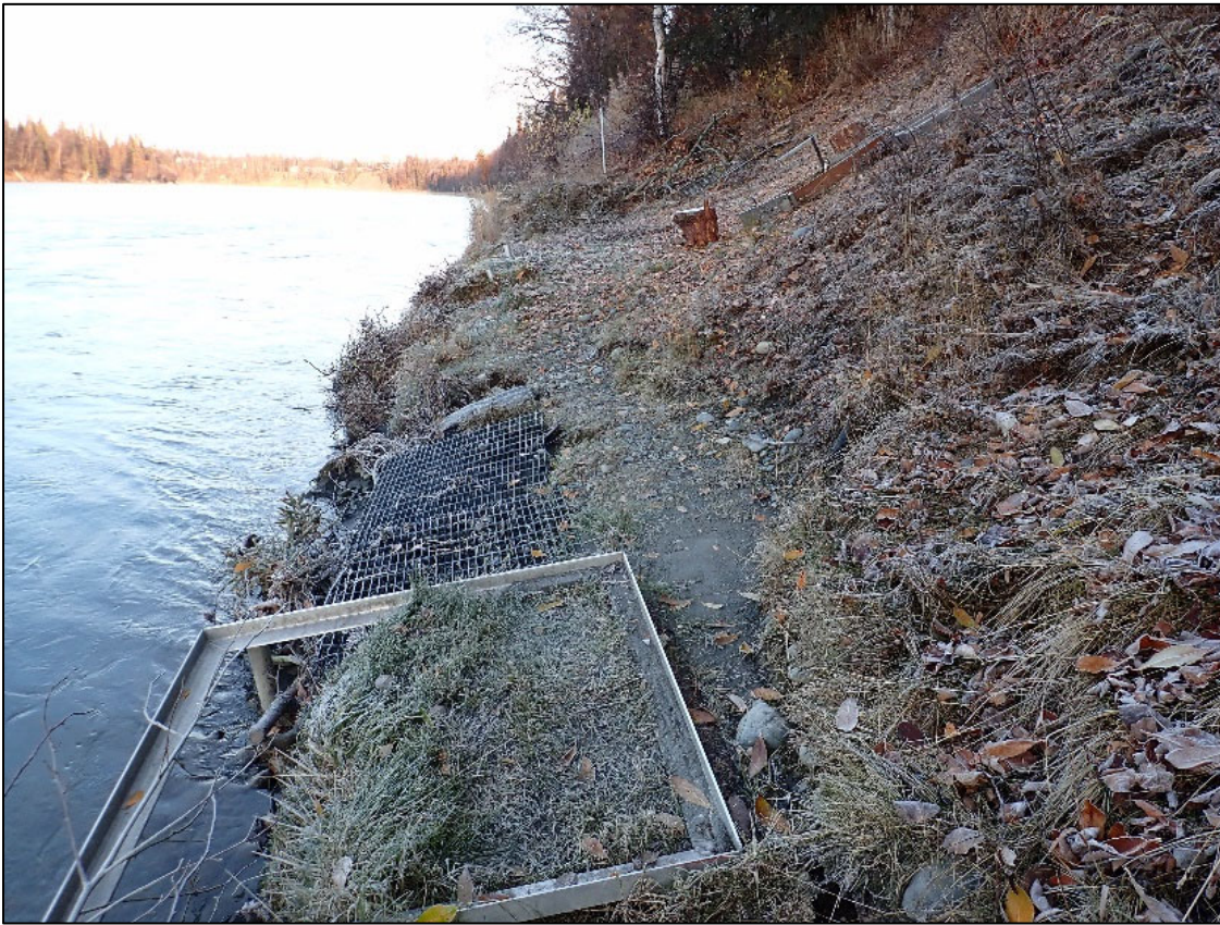
Figure 2. Looking downstream at a streambank where the riparian vegetation was removed and damaged from foot traffic causing accelerated erosion.
