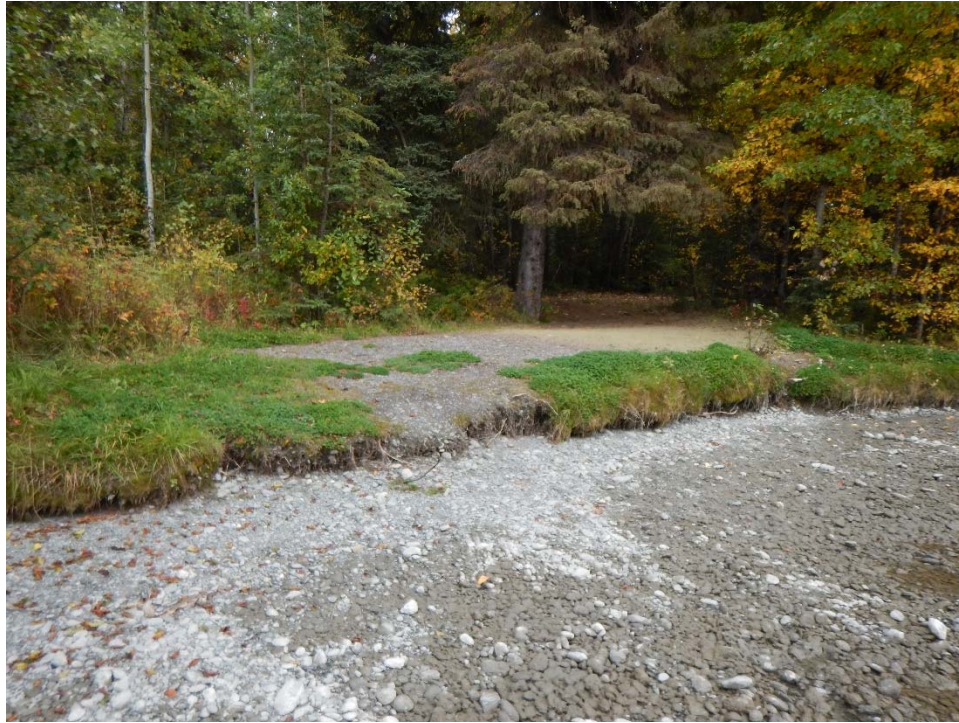
Figure 2 - Impacted Riverbank and Exposed Cable (September 18, 2018)
