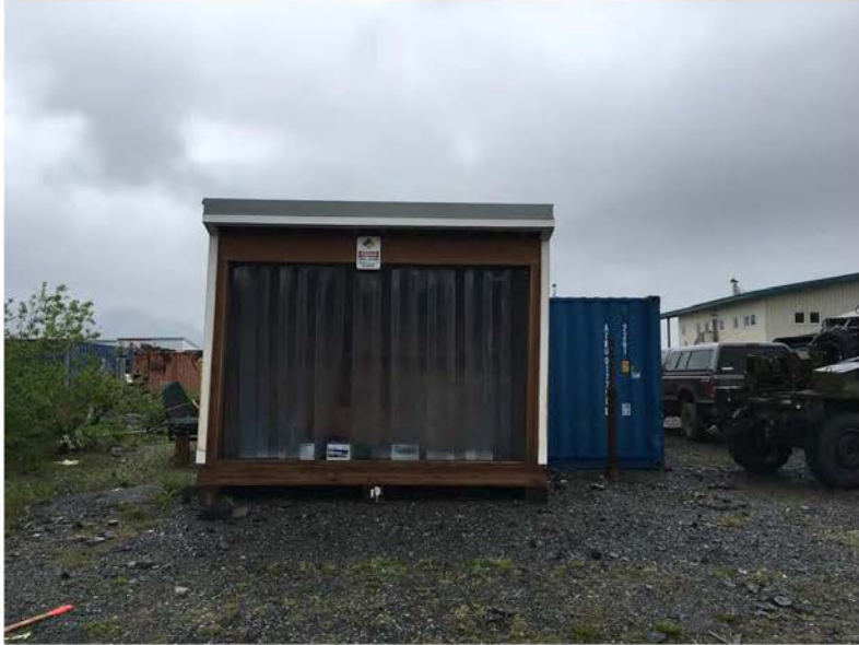
Lead Acid Battery Shed
