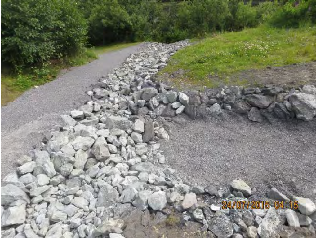
Re-constructed foot and vehicle access path, rip rap drainage ditch to prevent erosion of gravel and fine sediment, and sediment trap basin. July 2015.
