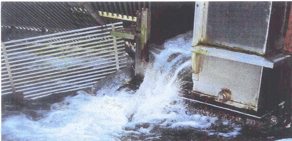
Figure 6. Photos of the third bypass entrance tank and diversion weir at Little Waterfall Creek, after 1995 modifications to improve salmon passage. Note pink salmon entering the entrance tank in the middle photo.
