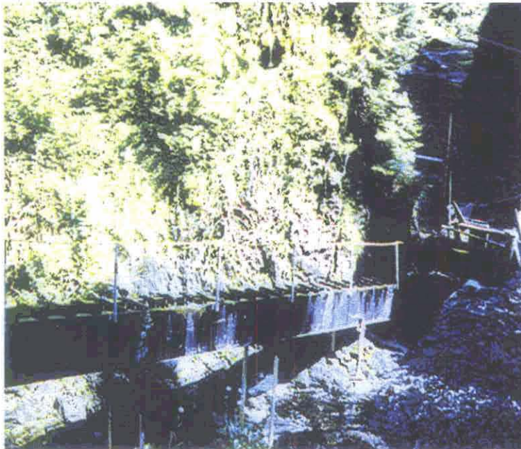
Figure 4. Photos of the most upstream bypass (third bypass) at Little Waterfall Creek, prior to 1995 modifications to improve salmon passage.
